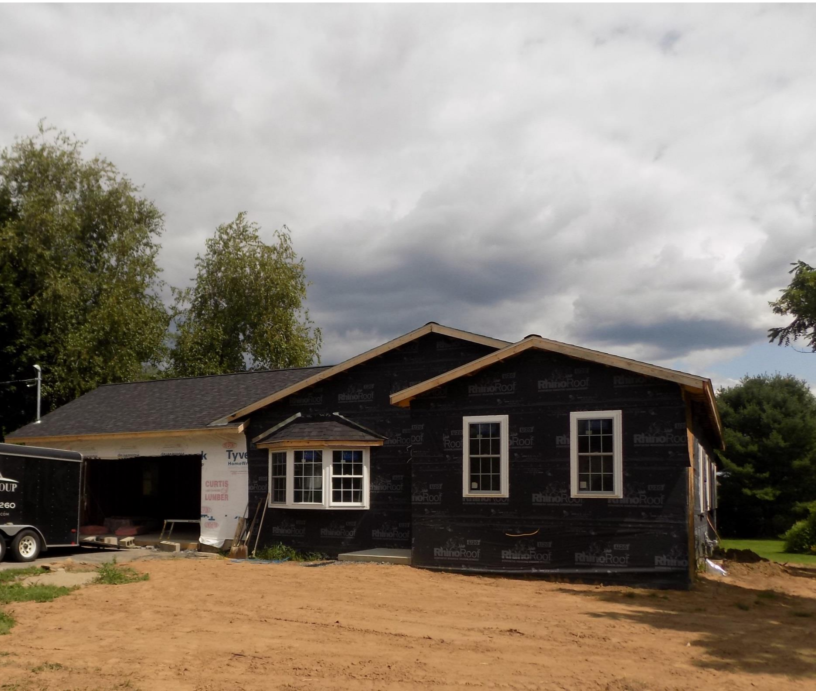
A property purchased from the Land Bank undergoes renovation in Bethlehem, NY.
