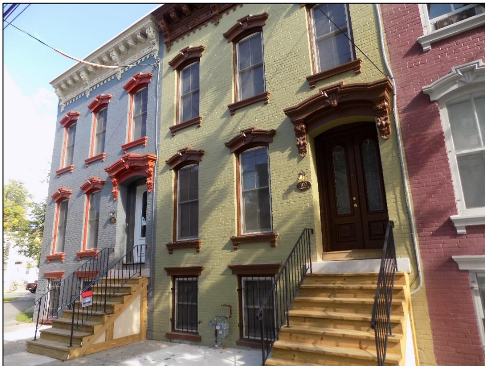
Two full rehabilitations completed in partnership with Habitat for Humanity Capital District on Lark Street in Albany. These homes will be sold to first time homebuyers.
