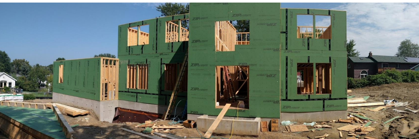
Construction of a new home is underway on a vacant lot purchased from the Land Bank in Colonie, NY.
